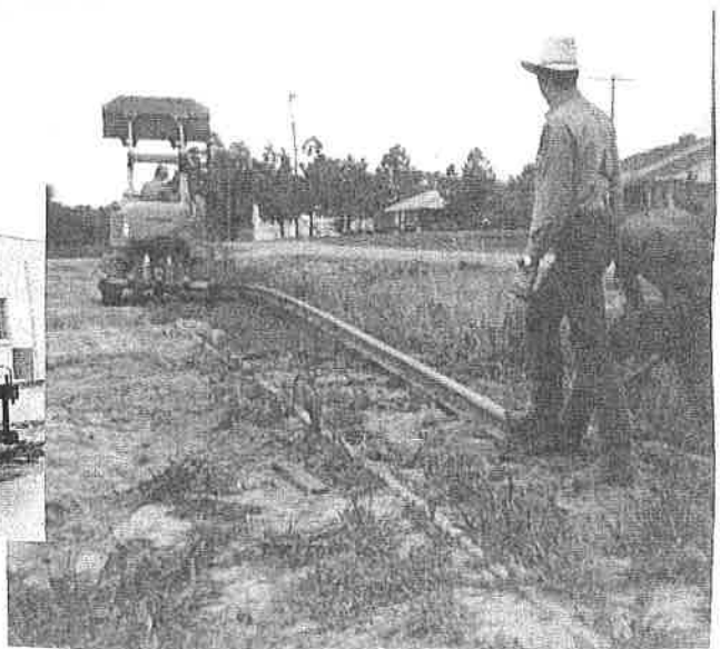
The tracks being removed from the town. The job was done by Powell and Allen Const.
